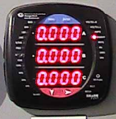
FEEDER 4C METERING
