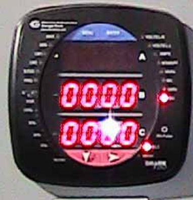
FEEDER 4A METERING
