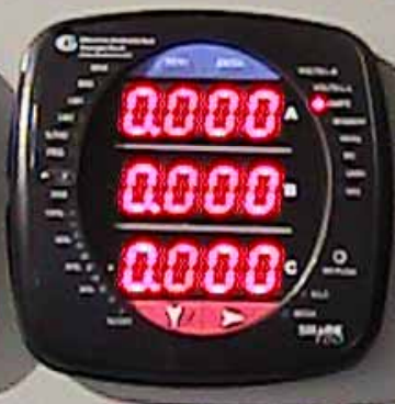
FEEDER 2B METERING
