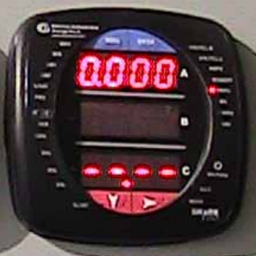
FEEDER 2C METERING
