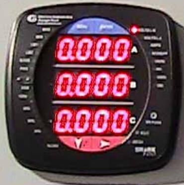
FEEDER 2A METERING
